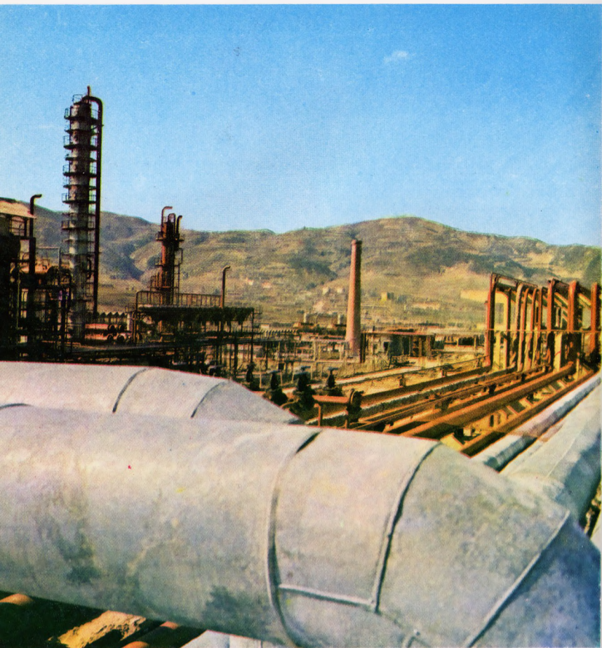
New deep oil processing plant.
